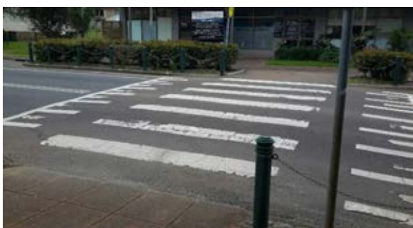
Non-compliant zebra crossing (no tactiles): ZC_00003
